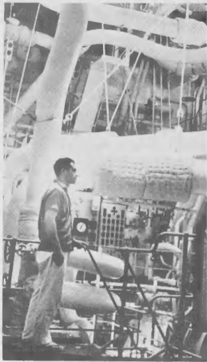
A MAZE of insulated steam lines face the visitor to the tanker's engine room.
